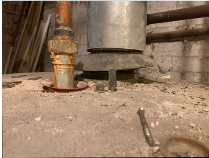
poor draft diverter
