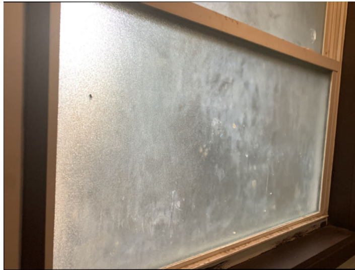
failed seal 3E
