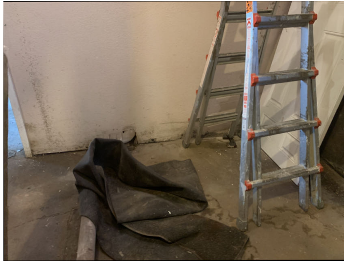
mold stains in basement
