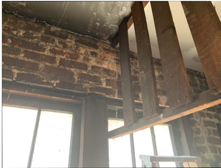
efflorescence - courtyard wall
