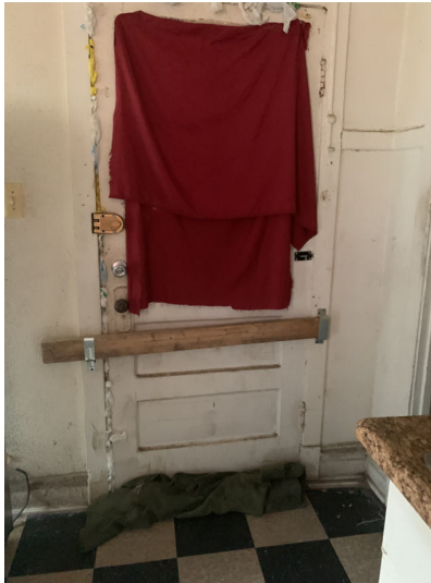
2W blocked door
