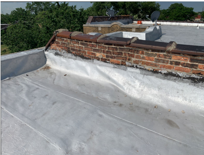
poor termination bar
