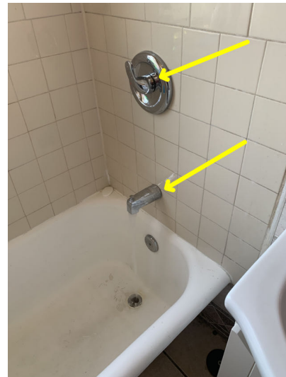
3E2 loose with gaps
