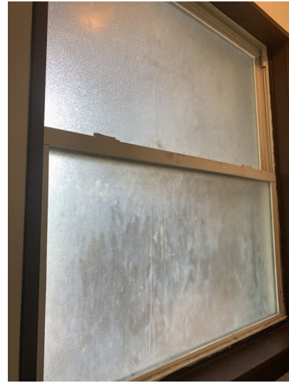
failed seal hall 3W
