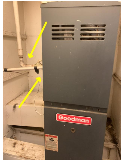
3W older Missing drip leg on gas
