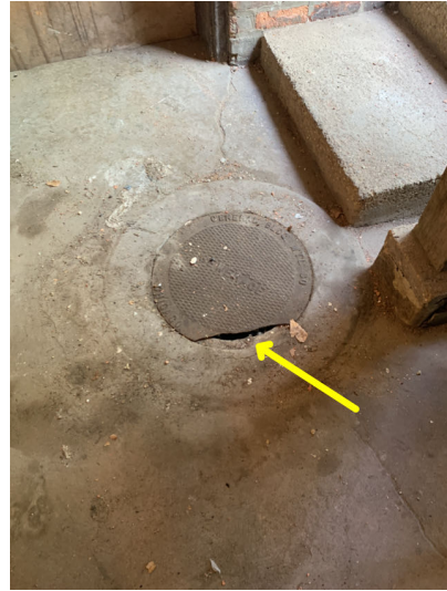
rear catch basin
