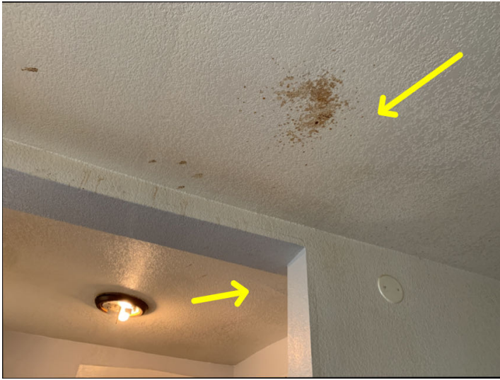
1W leaking and stained
