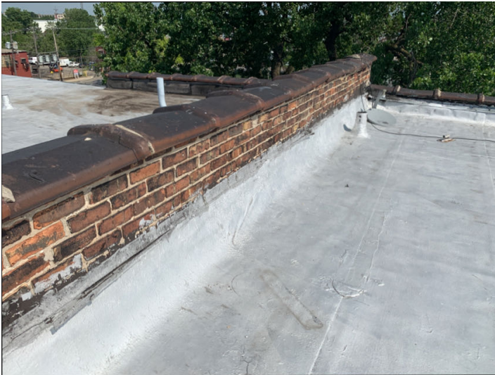
poor termination bar
