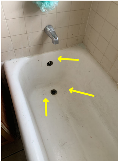
3W Missing overflow and damage
