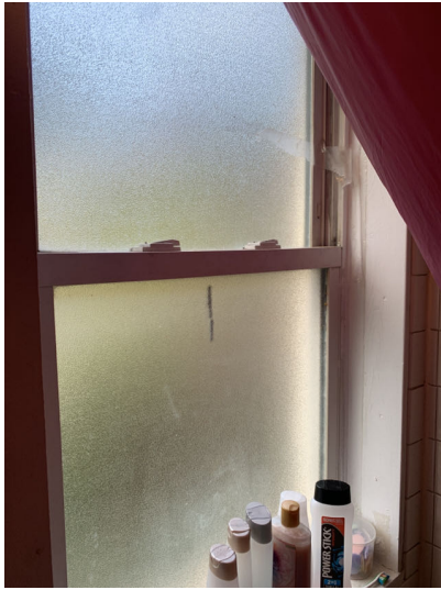
1E Failed seal
